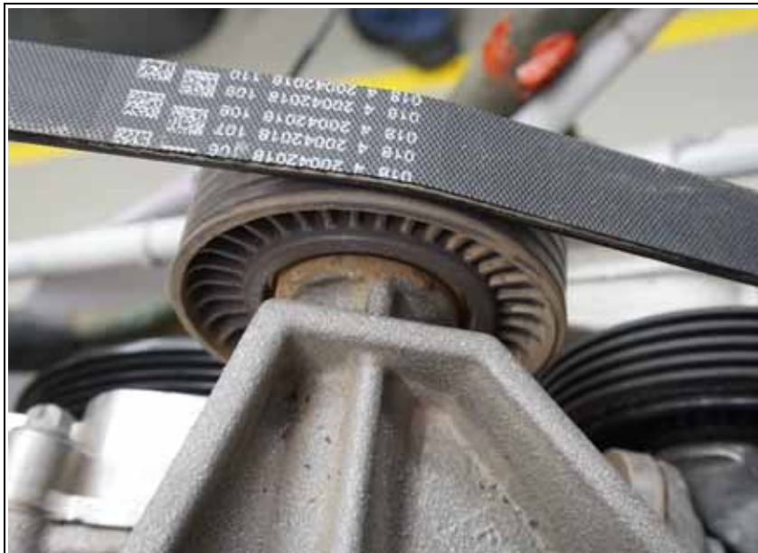
Fig. 6.60 Inspecting the V-Ribbed Belt Pulleys OK
